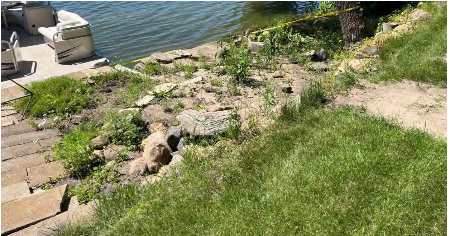
Bottom of slope/gully where it outlets into lake
